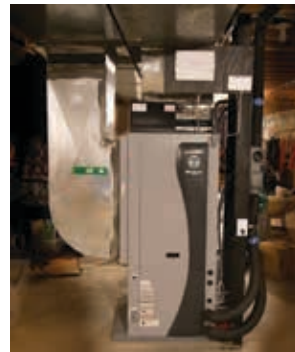
An example of in-building geothermal heat pump equipment
